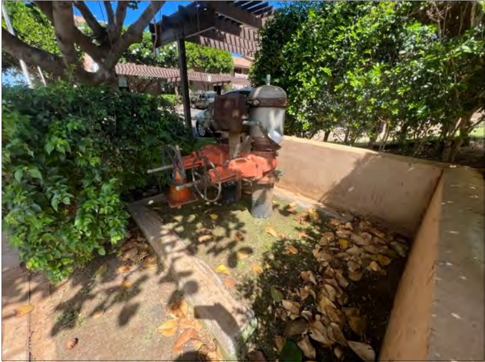
Fire Hydrant DCDA Backflow Preventer
