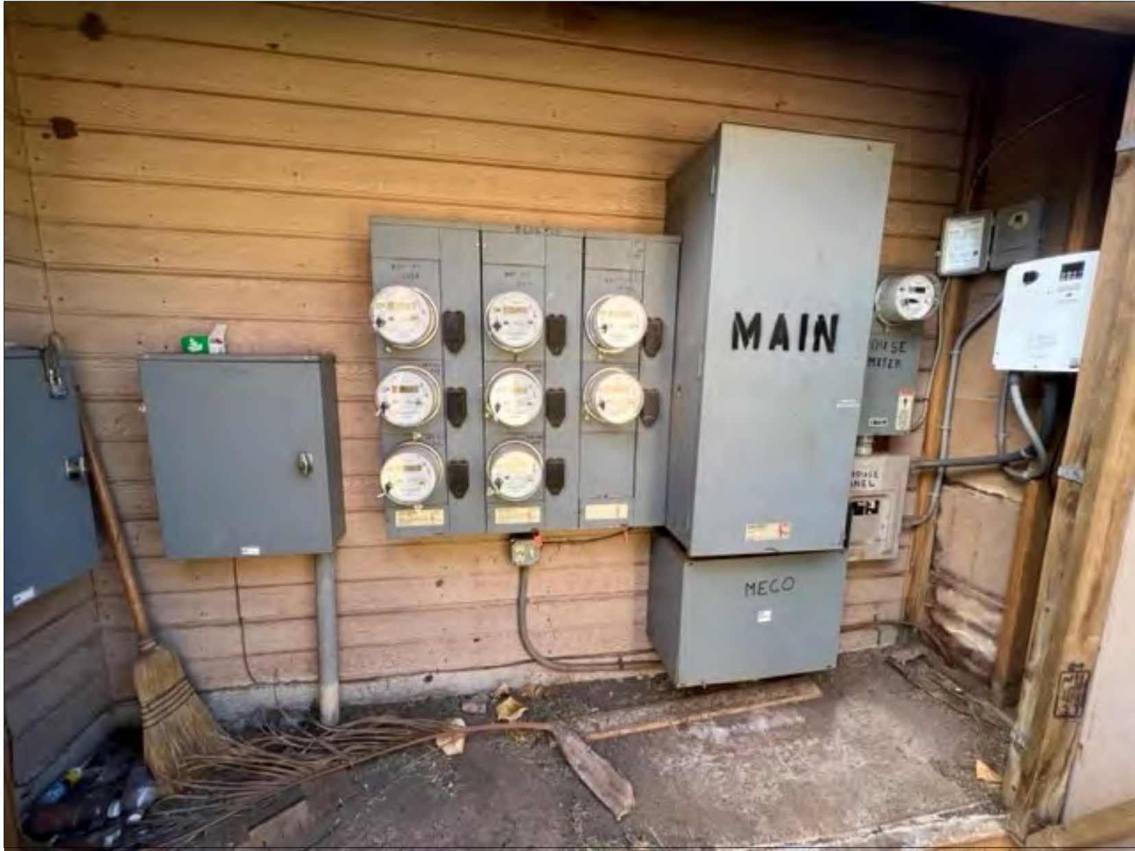
Electrical Socket Meter Panels, Main Connection Box, House Meter, Timers and Well Control Panel
