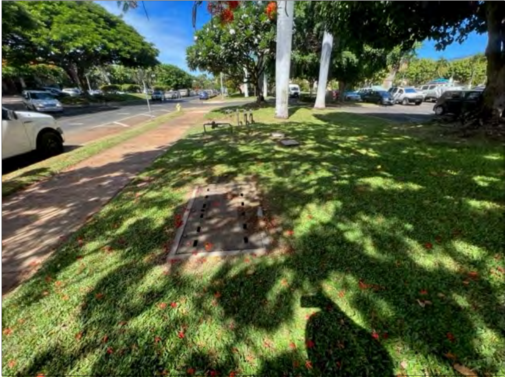
Irrigation and Domestic Water Backflow Preventers
